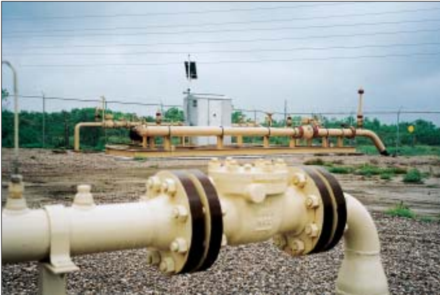
TXCO's Maverick-Dimmit Pipeline Ltd. can move as much as 12 MMcfd of gas to the Mexican market through this sales point with Tidelands Oil & Gas Corp. east of Eagle Pass, Texas. The 12-inch line entered service in late 2003.
